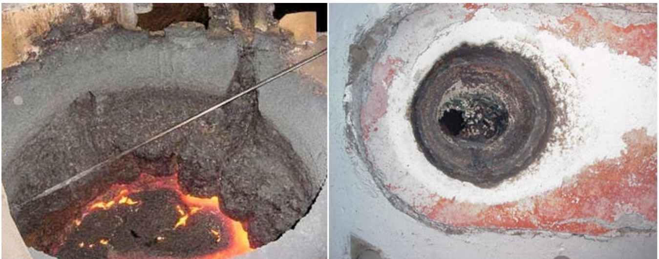
Figure 2a, (left): Severe slag build-up in the upper case of a channel furnace.
